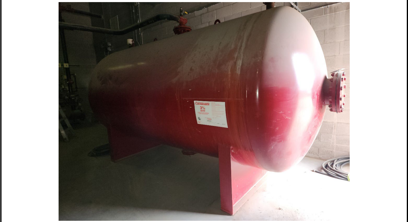
Location/Description: AOC 25: Bombardier Building X – 2,400-gallon AFFF concentrate tank for overhead FSS
