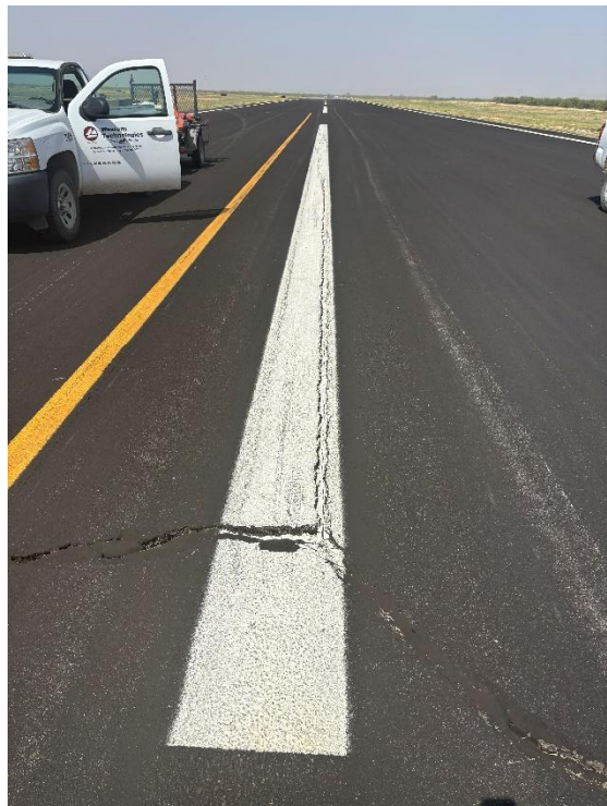
L2. View west with Crack U3 in foreground.
